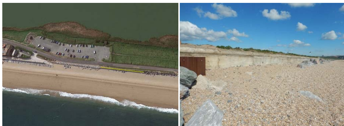
Figure 4-2 Concrete seawall; Left - location of works indicated by yellow line and Right – photograph of the seawall Source: Left - (© 2015 Google Earth) and Right – photograph taken during condition assessment on 27th April 2017, looking north-east
